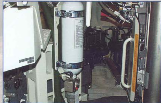
Fire suppression system
